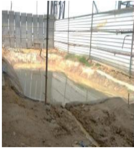
Figure 14: Sedimentation tank connected via soil erosion channel
