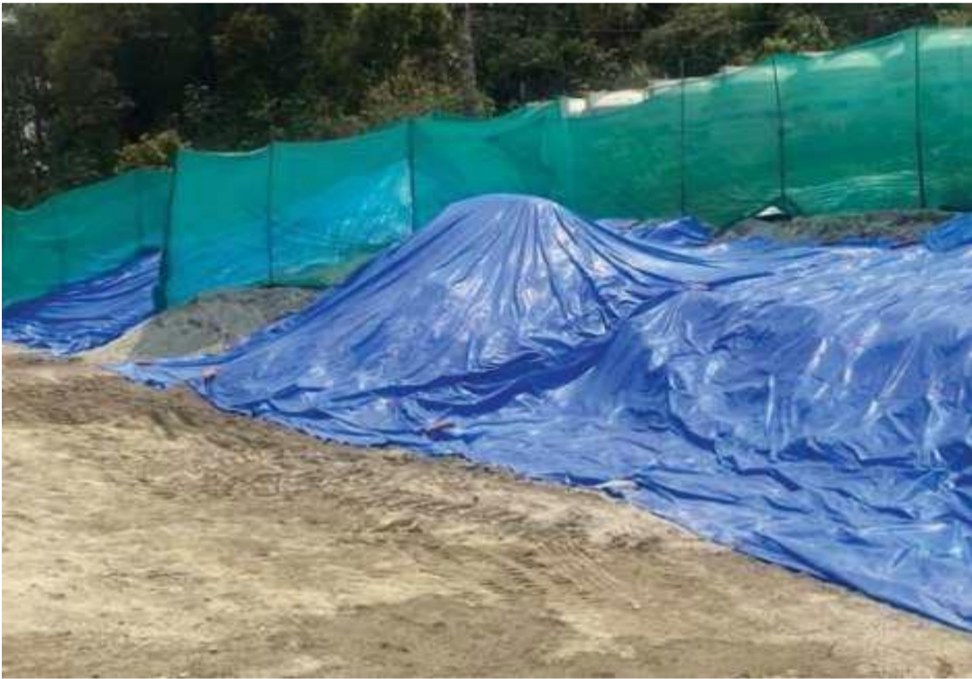
Figure 7: A good example of covered fine aggregates
