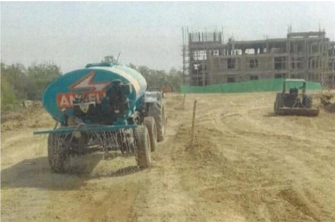
Figure 8: A good example of water sprinkling of excavated earth during construction using STP treated water
