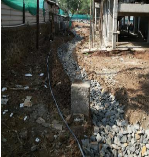
Figure 13: Soil erosion channel with gravel belt
