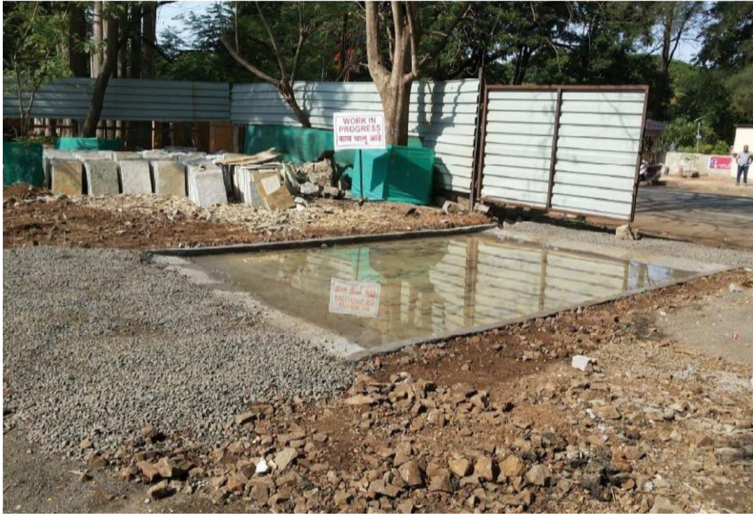
Figure 5: A good example of a wheel washing facility at all entry and exit points of the site.
