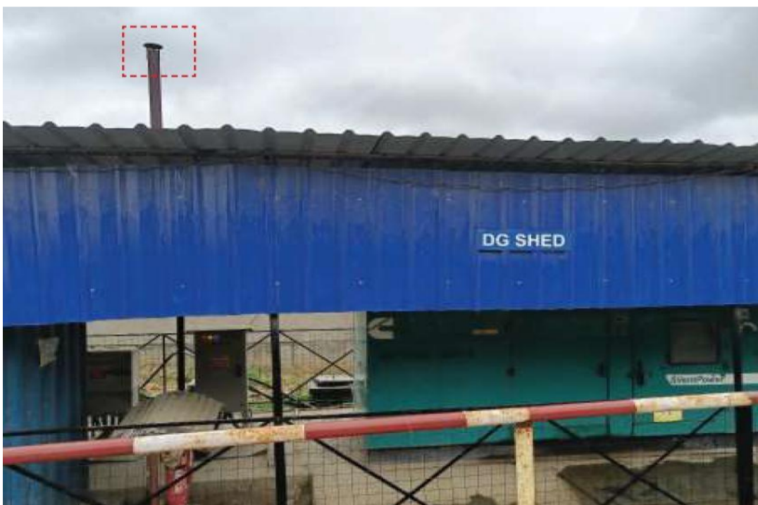
Figure 6: A good example of DG set with proper chimney stack height
